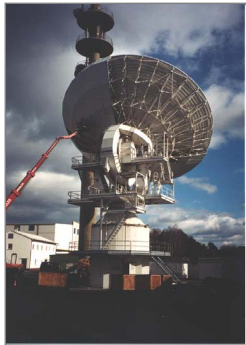
Walton Field Technician installing a Walton Hot Air De-icing System on a 18-meter Antenna
