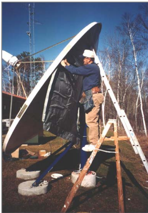
Walton Field Technician removing a competitor's Anti-icing system prior to installing a Walton System
